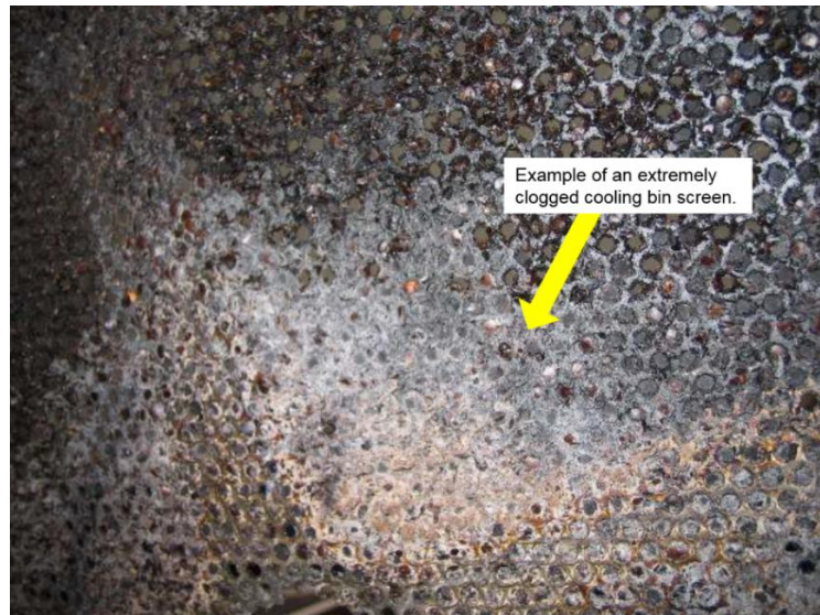
Dirty Cooling Bin Screen
