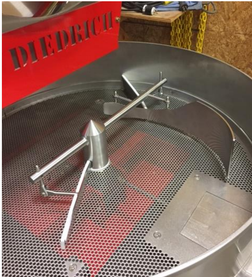
Example of a Clean IR-5 & IR-12 Cooling Bin Screen
